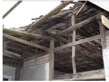
6. 桁架斷裂損壞*
